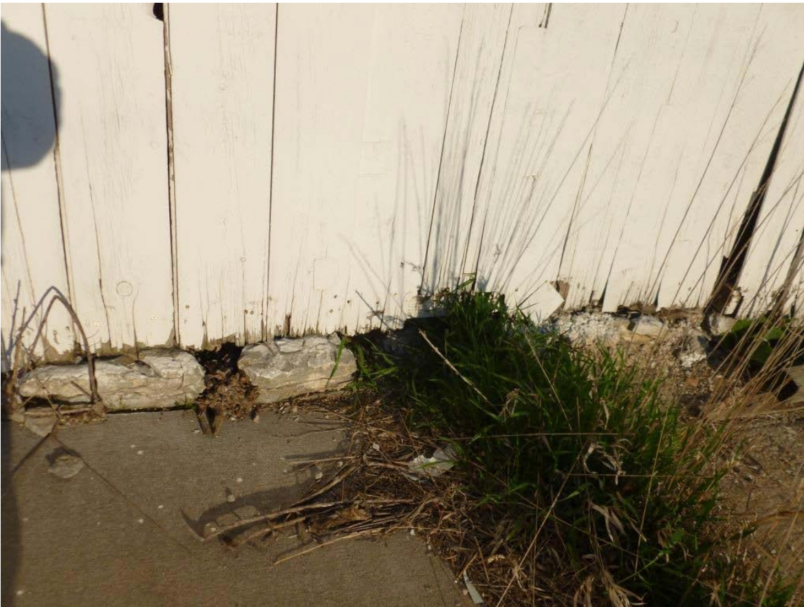
foundation, siding in need of repair, weeds
