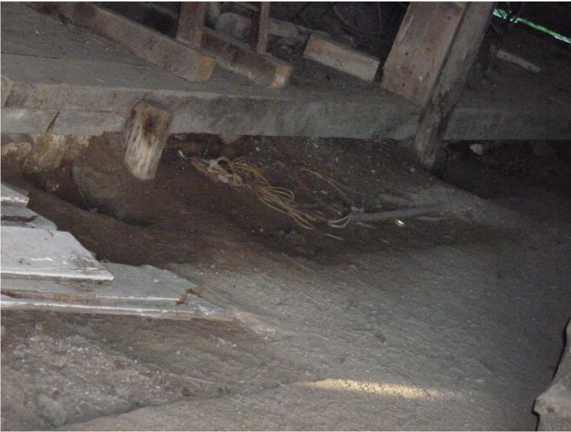
Vermin holes in foundation
