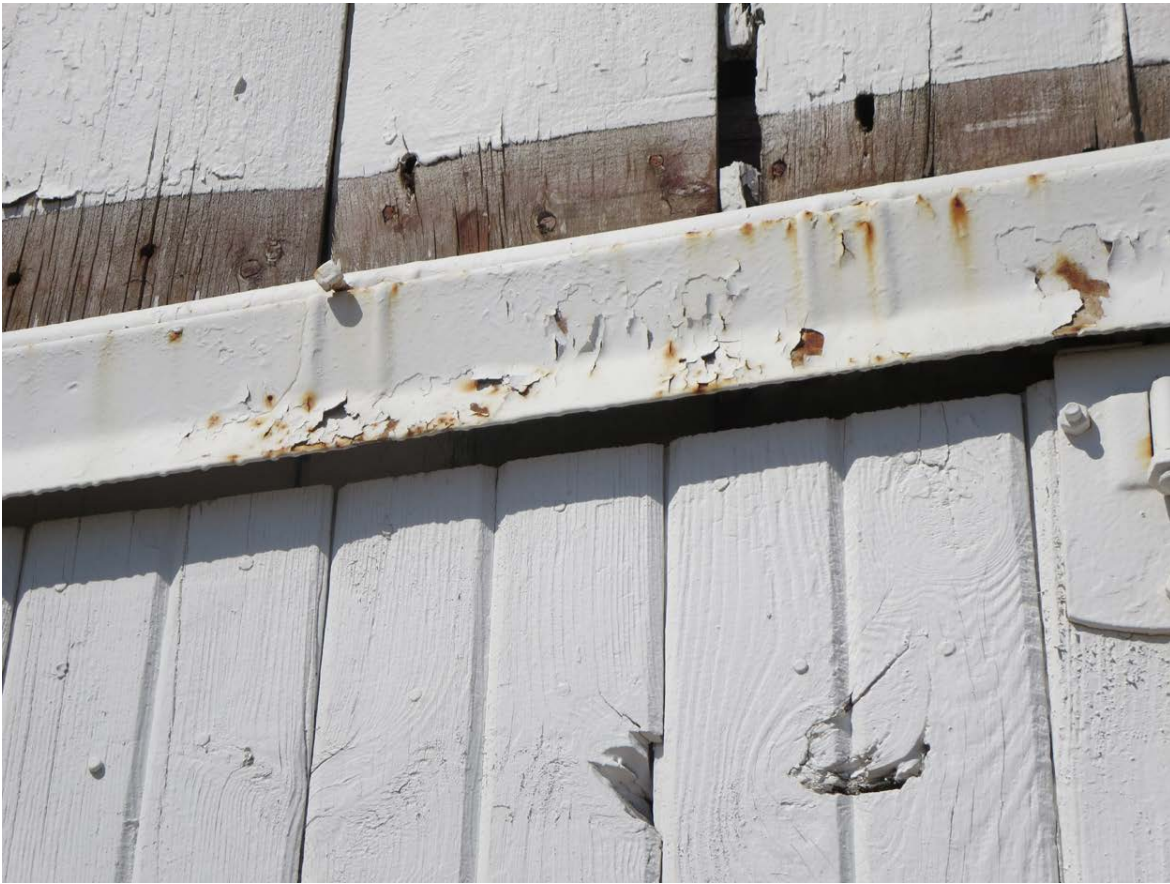
Misaligned sliding door
