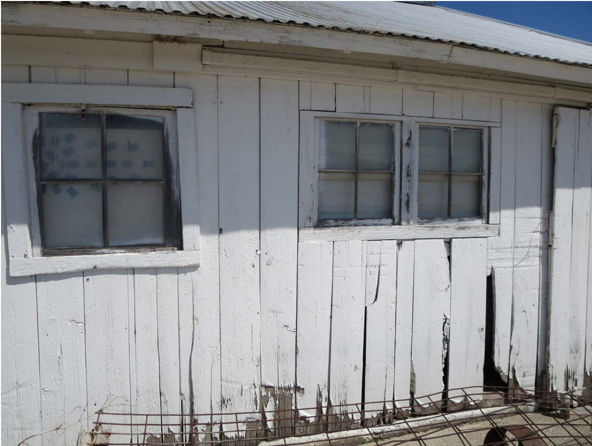
Windows, siding in need of repair
