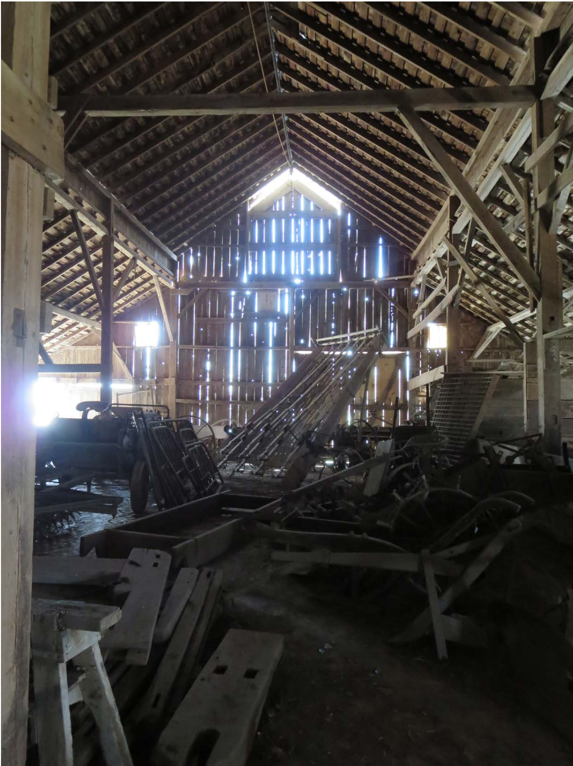
View of missing cross beams
